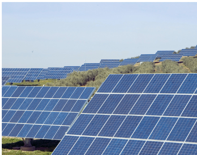
5.4 MW solar plant in Alcaudete, Jaen (Spain)
